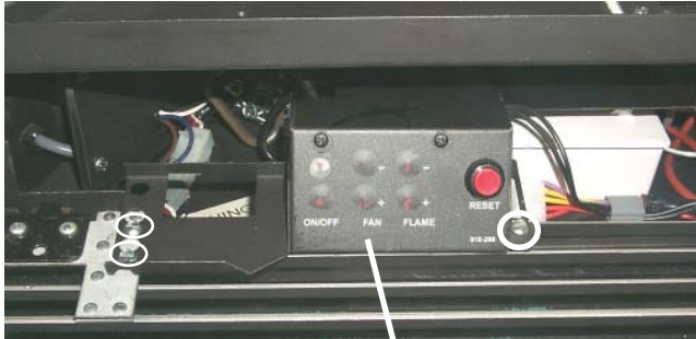
Manual Control Box
